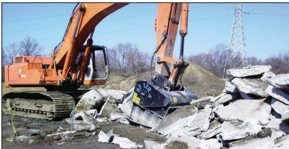
This pile of debris is being recycled on site, saving hauling and tipping fees.
