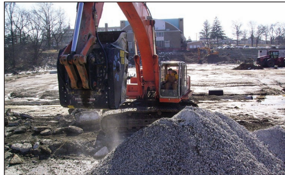
Art Anderson, Inc. was contracted to demolish stadium with cast in place bleachers (left).
